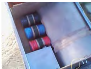
Fig. 30. "Twister" by Tariel Kapanadze using a three-phase "zero-transformer".
